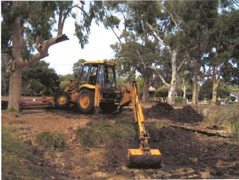
The excavator at work. The water-rat's nests and tunnels were under the stone bridge on the right.
